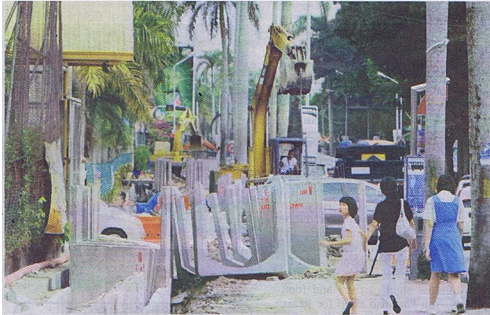
Widening stretch: The upgrading works on Jalan Gottlieb and Jalan Bagan Jermal have begun.
