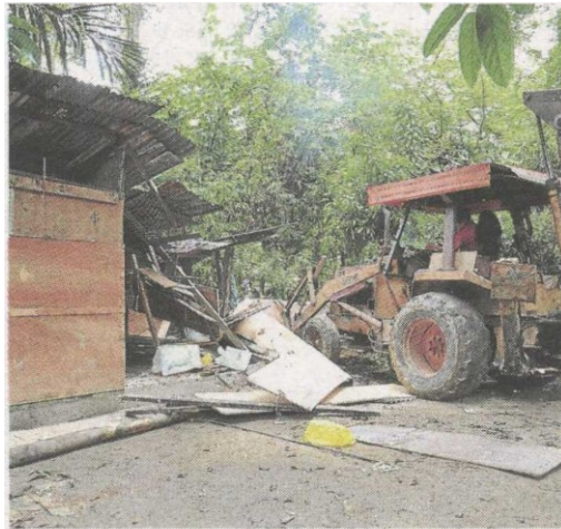
Knocked down: The wheeldozer moving in to demolish the shed built by Cheong, which FRIM claims was built in April 2013 despite an eviction notice sent in July last year.
