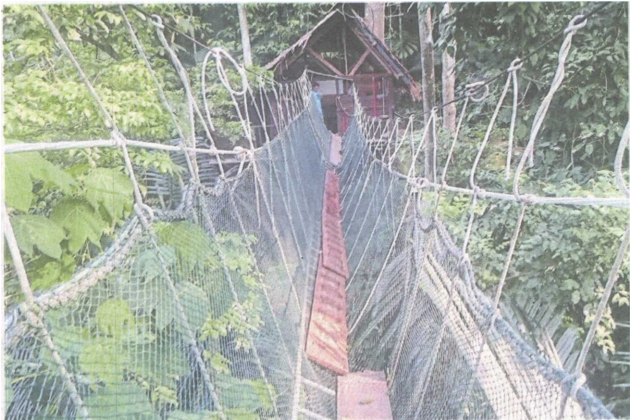
The FRIM canopy walkway that was damaged after a recent thunderstorm.
