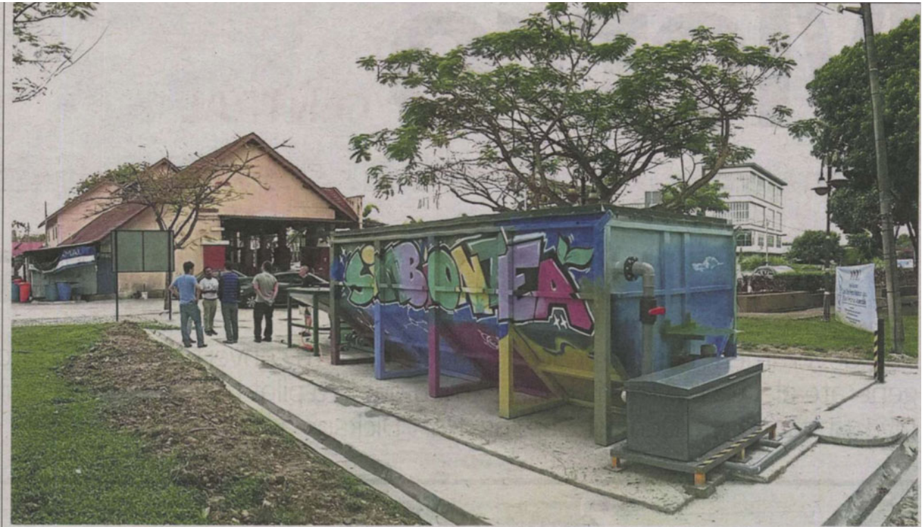
The anaerobic digester system installed beside the Dengkil Food Court
